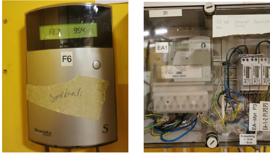
Fig.4 The flow meter and electricity energy meter
