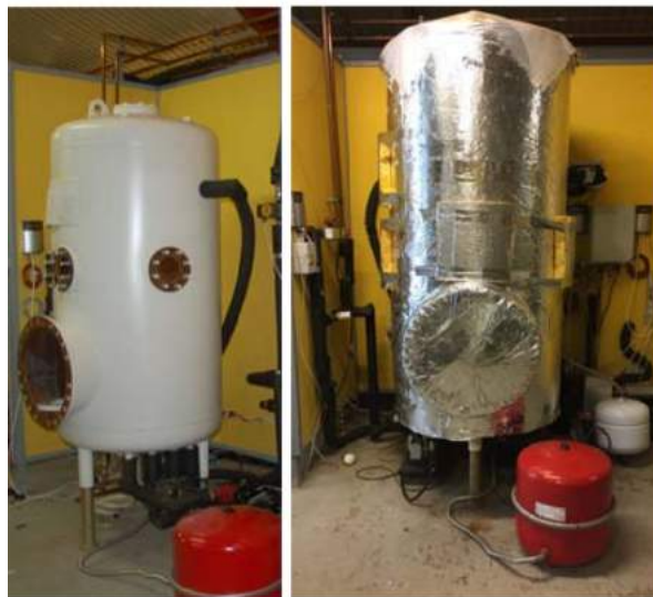
Figure 1.4: Pictures of storage tank-in-tank.
