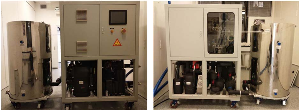
Figure 3. The ice-source heat pump developed for the solar heating application.
