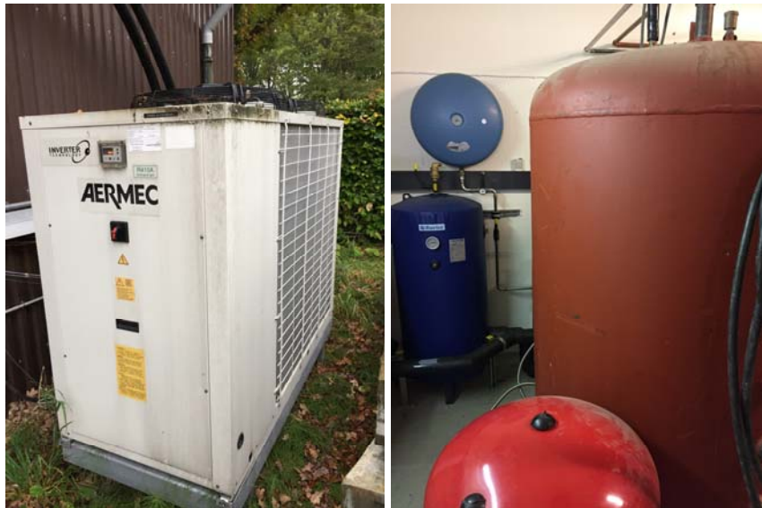
Figure 10. Cooling system and heat sink in the test facility.
