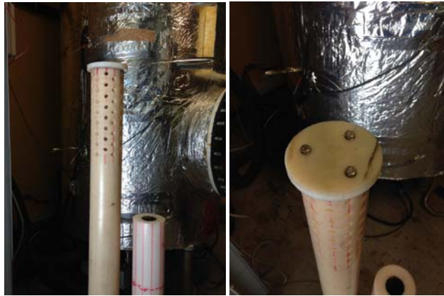
Figure 5. Pictures of the two pipes used to charge the storage tank with space heating water.
