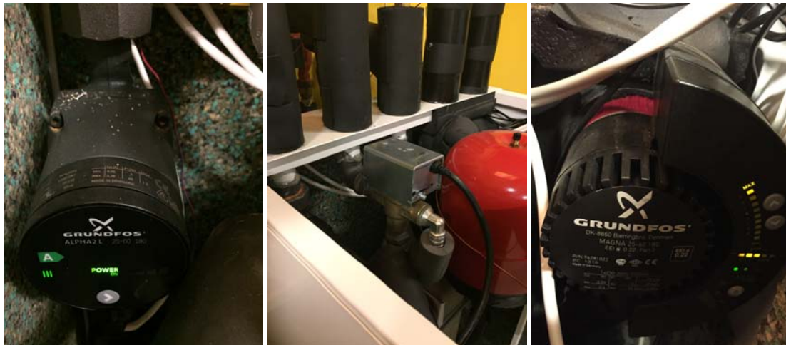
Figure 9. The two pumps and the 3-way motor valve in the heat pump.
