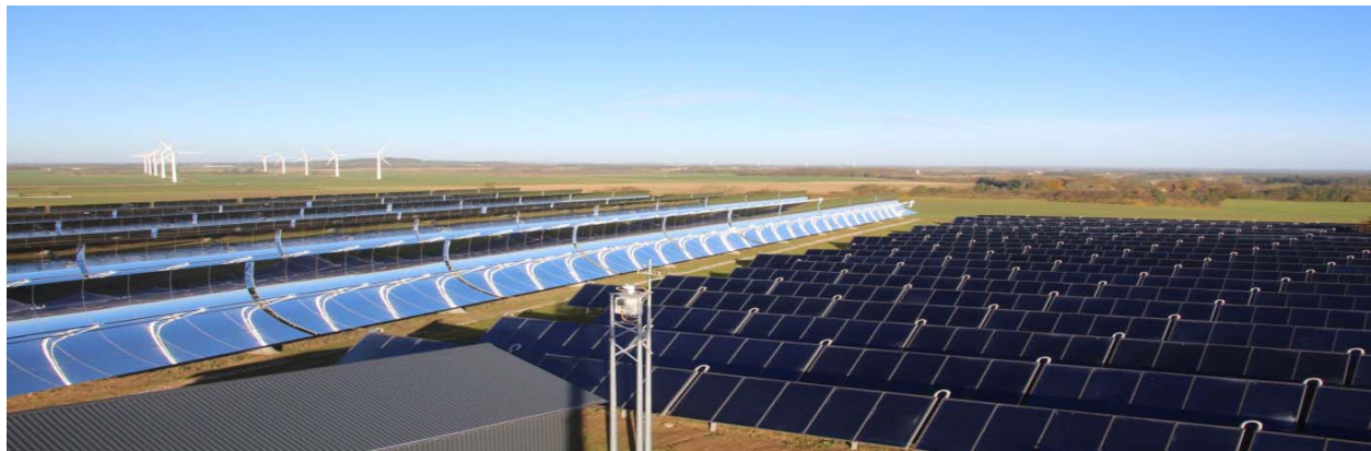
Fig. 18: solar collector arrays in Tårs solar heating plant
