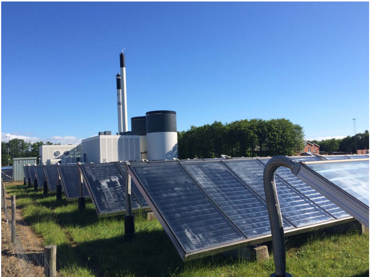
Fig. 12: Solar collector arrays in Sæby solar heating plants
