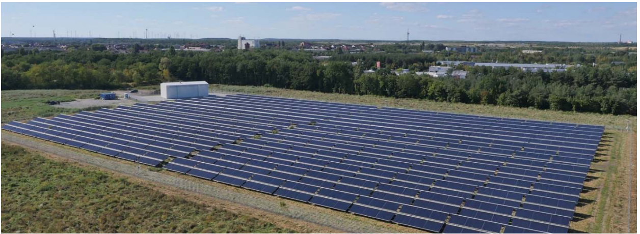
Fig. 9: Solar district heating for 3,000 households in the German town of Senftenberg [10]
