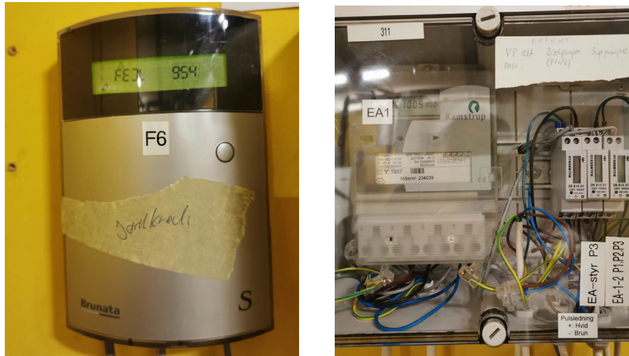
Fig.4 The flow meter and electricity energy meter
