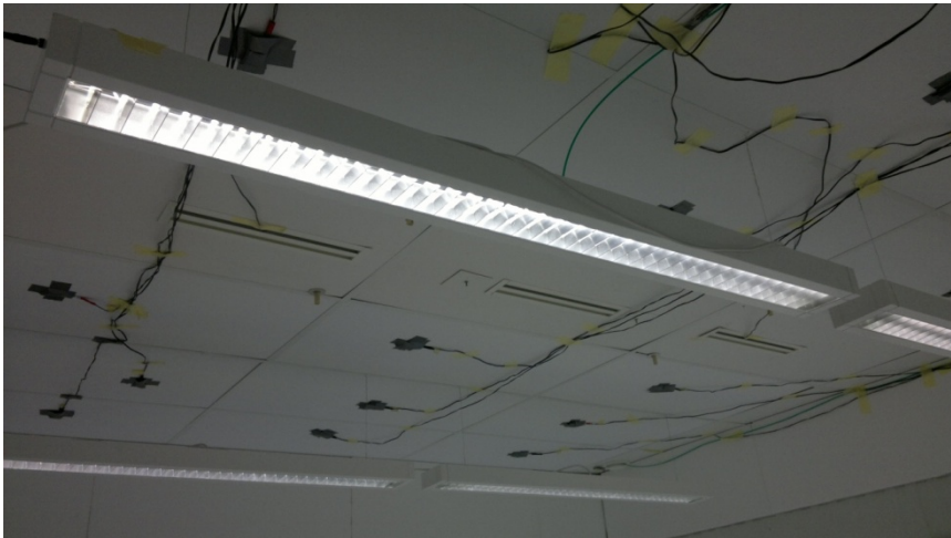
Figure 3.11: Chilled ceiling radiant panels with sensors attached and linear slot diffusers in the middle row.
