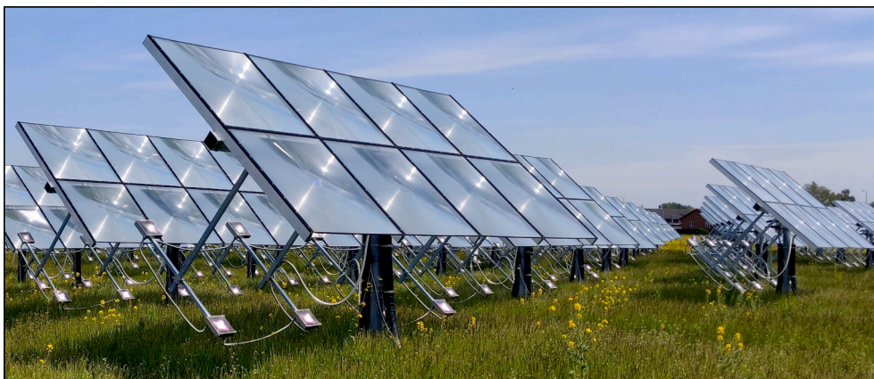
Fig. 1. Photo of the Fresnel lens solar collector field in Lendemarke, Denmark during operation. The white spot in the receiver boxes is the focus point of the lenses. The photo was taken when the field was inaugurated and the pipes have since been insulated.
