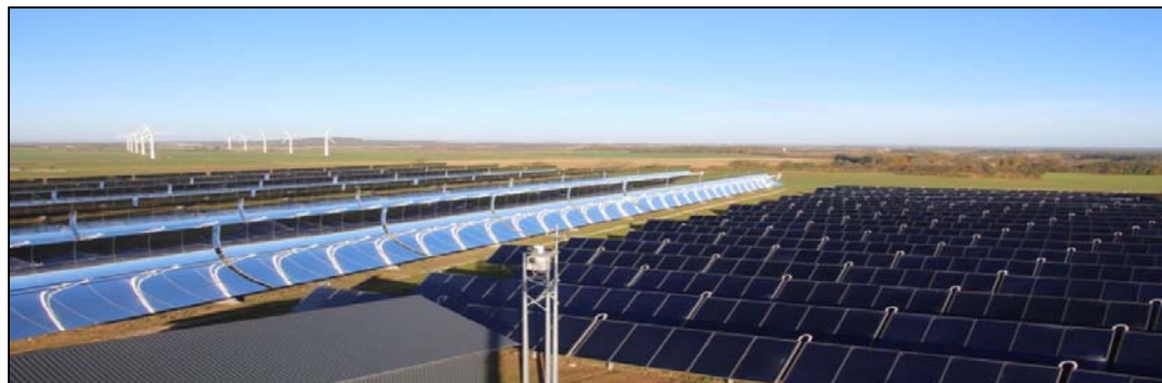
Fig. 2: solar collector arrays in Tårs solar heating plant.
